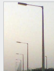
Street Light Poles
